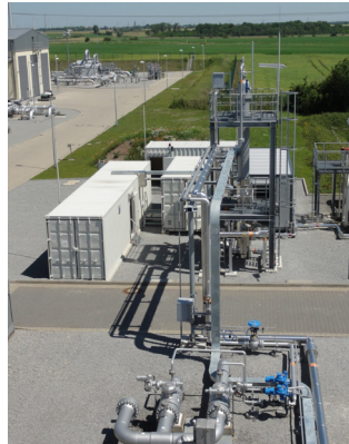
Pilot plant for dehydration of natural gas with membranes (UGS Staßfurt).
